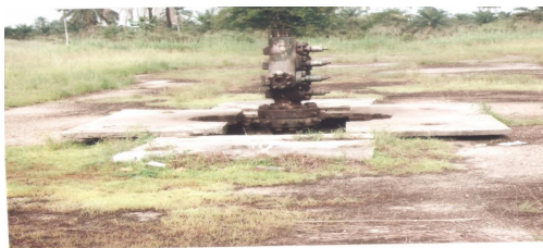
FIGURE 2 | Destroyed vegetation at odagwa spill site.
